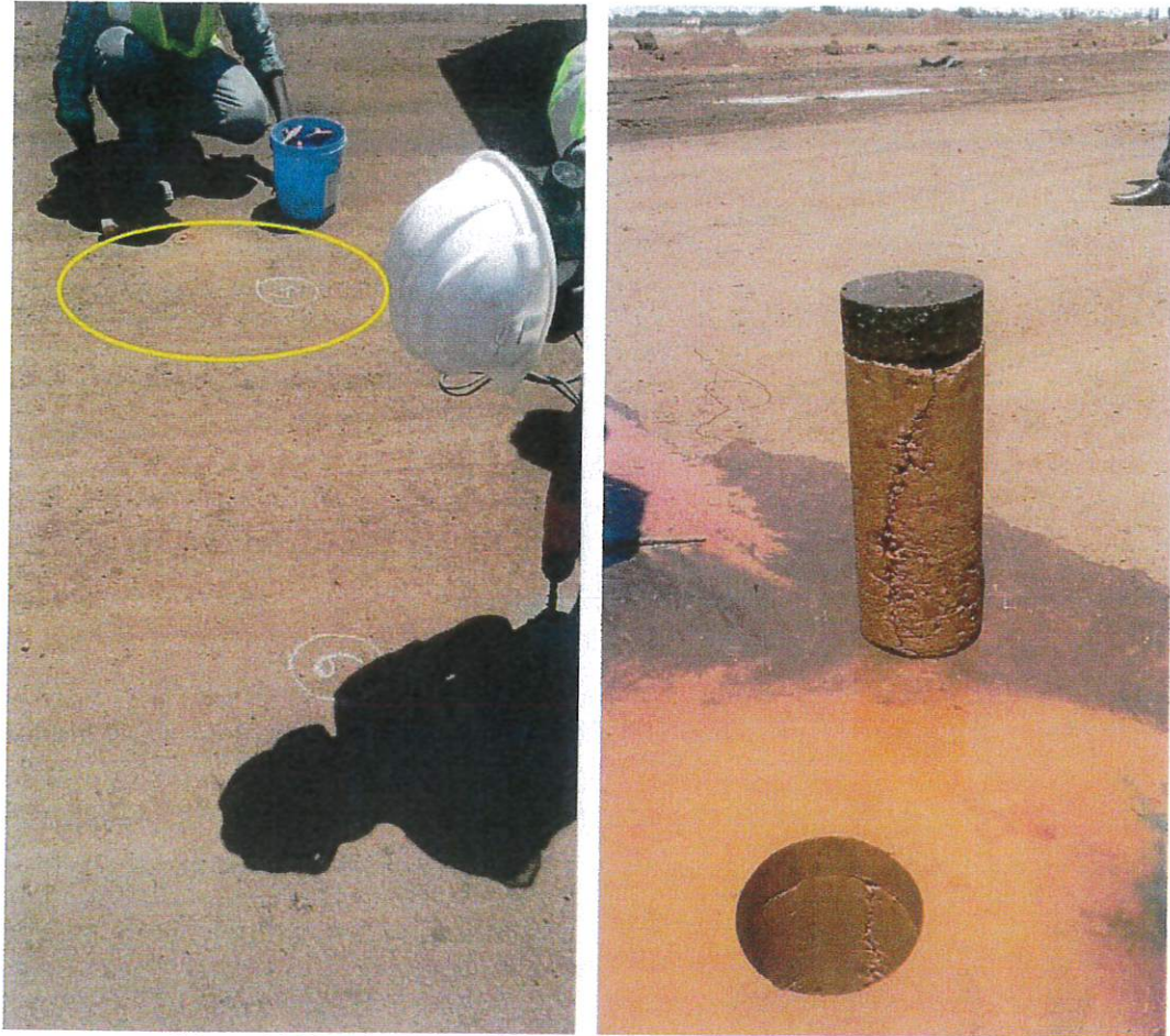
Photo 23 Depth of Crack propagation on Stabilized Pavement
