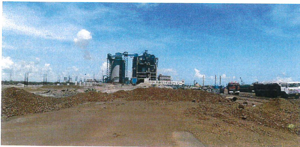
Photo 3 Original soil replaced with Murrum soil up to 1m depth from the EGL
